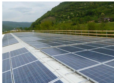
Location: Cuneo, Italy Project Type: Roof Top Project Scale: 1.8 MWp
